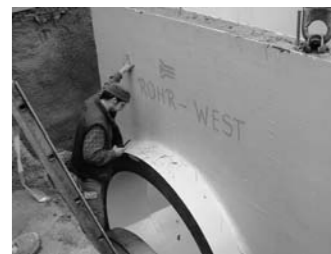
After the pipe couplings have been pushed onto the ends of the pipe, the concrete chamber is lowered in alignment with the pipe axis.
