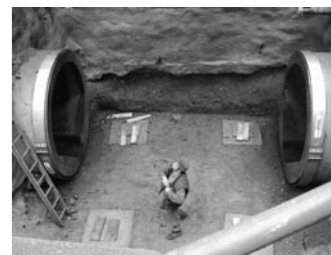
A section of the sewer pipe has been removed, ready for installation of the flow retarder.
